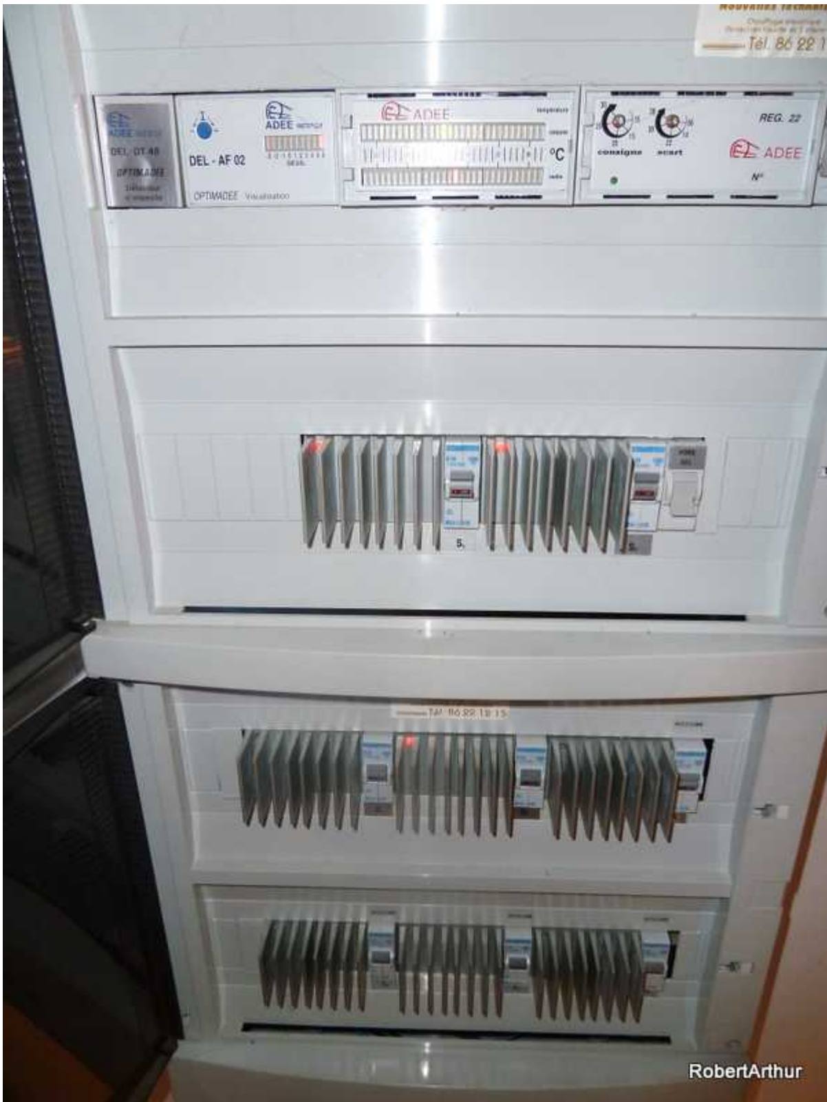
King of the hill délestage unit. We had almost 24 kW of accumulateurs and convecteurs. On a “simple” 12 kVA supply in single-phase.
